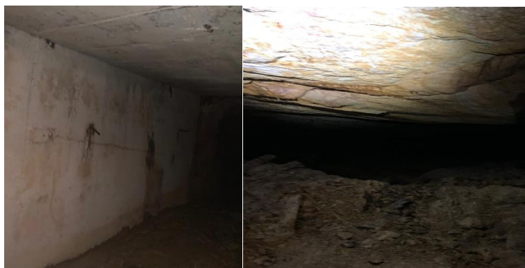
Image 5: Good conditions reported of the Qala Adit shaft infrastructure (left) and the K9A hanging wall (right)
