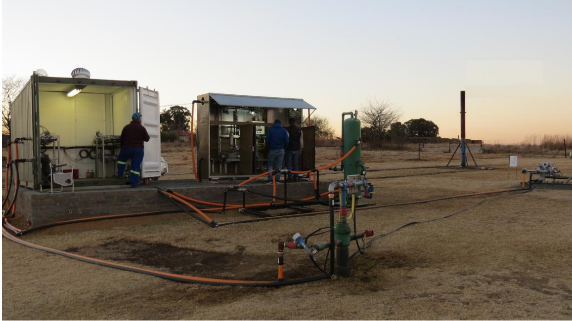
Figure 4 – Gas separator and well head equipment on Well KA-03PTR
