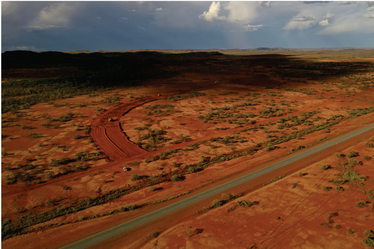
Figure 2: Commencement of Construction of Haul Road at Intersection to Public Nanutarra Road (foreground)
