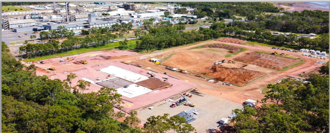
Aerial overview of HPA First Project Site, Gladstone – showing civil construction progress on left hand side.
