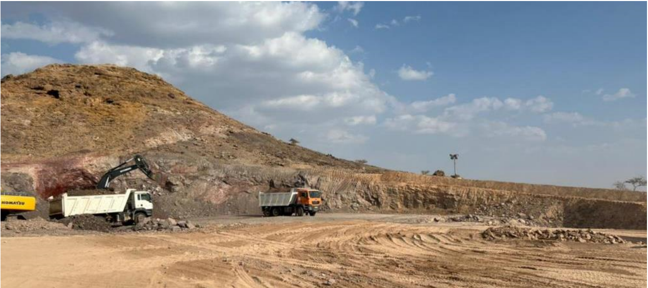
First cut mining activities and overburden and limited oxide copper ore removal
