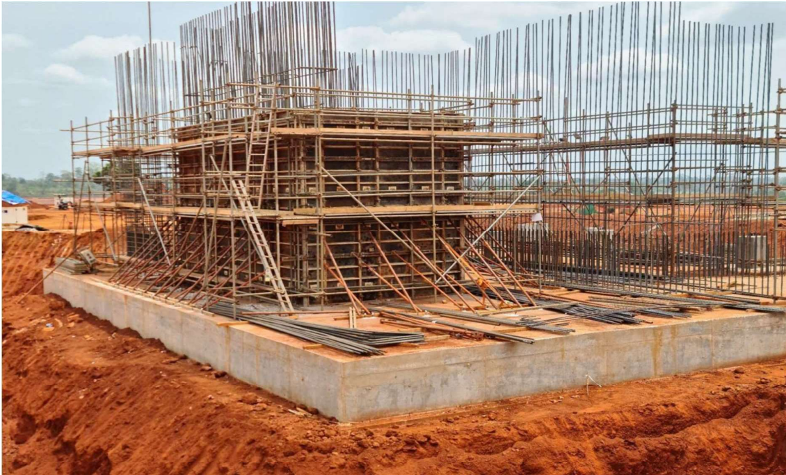
Figure 7: Abujar Gold Mine SAG Mill Free Bearing Core Walls Reinforcement and Formworks in progress
