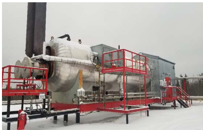
Large Treater on Red Earth Asset
