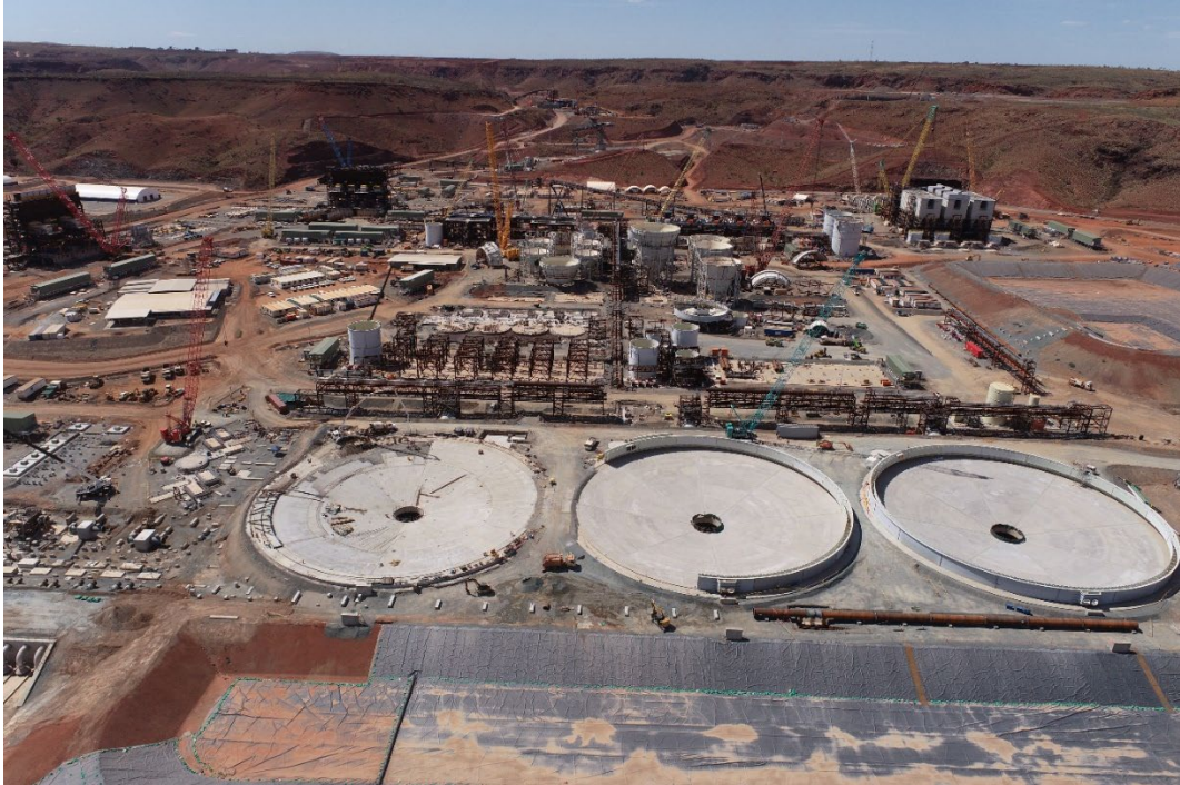
Iron Bridge Magnetite Project - Wet Processing Plant
