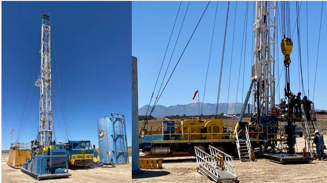
Work-over rig on the Jesse#1A well site in San Juan County, SE Utah, with the Abajo mountains in the background
