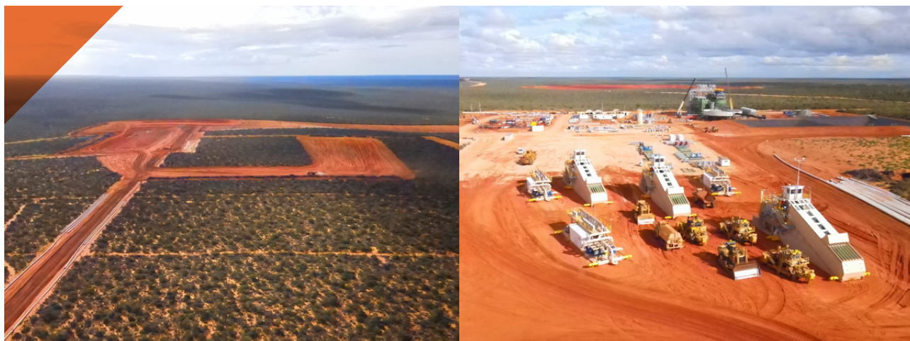
FIGURE 8: DEVELOPMENT OF OPEN MINE PITS & THREE DOZER MINING UNITS (DMU'S) READY TO BE MOVED INTO POSITION FOR MINING FIRST ORE
