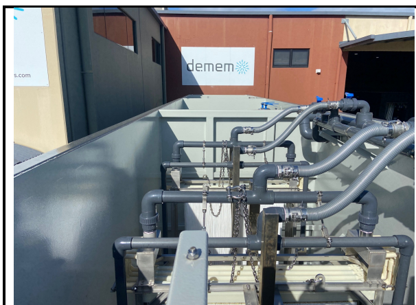
De.mem containerized waste water treatment system (1)
