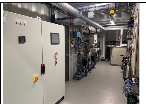
De.mem containerized waste water treatment system (2)
