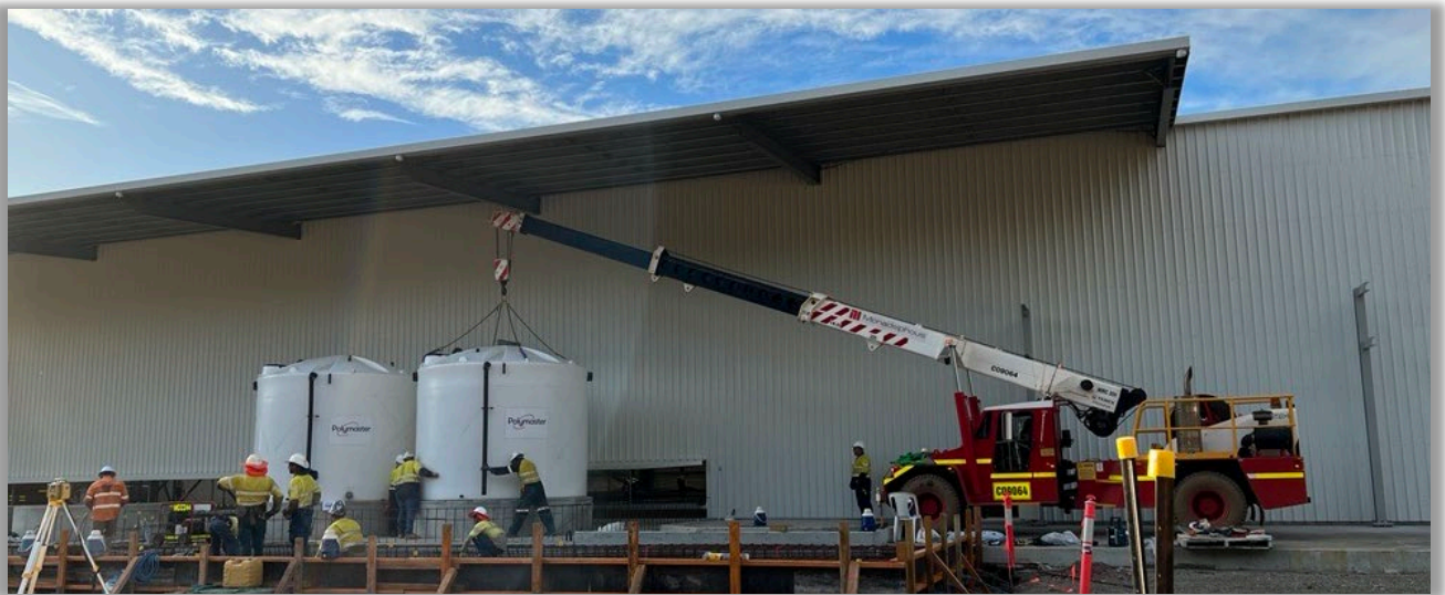
Installation of PPF reagent tanks
