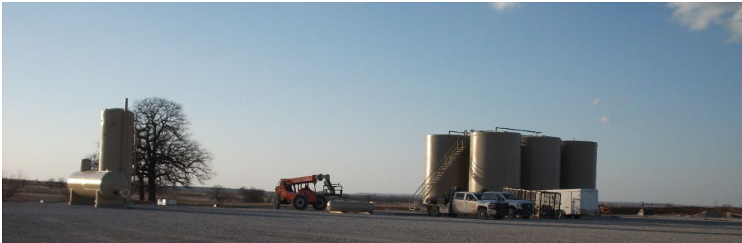
Figure 4. Rangers tank battery and separators
