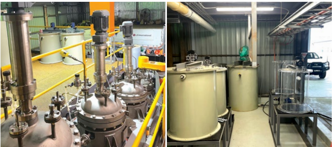
Figure 4 – Demonstration Plant. Left: Iron oxidation and precipitation circuit. Right: Installation of iron polishing and MHP precipitation circuits.
