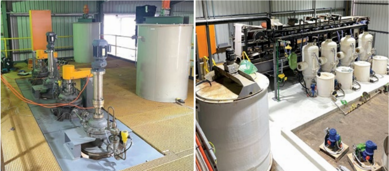
Figure 3 – Demonstration Plant. Left: Horizontal vacuum filter belt. Right: Pressure oxidation leach circuit.
