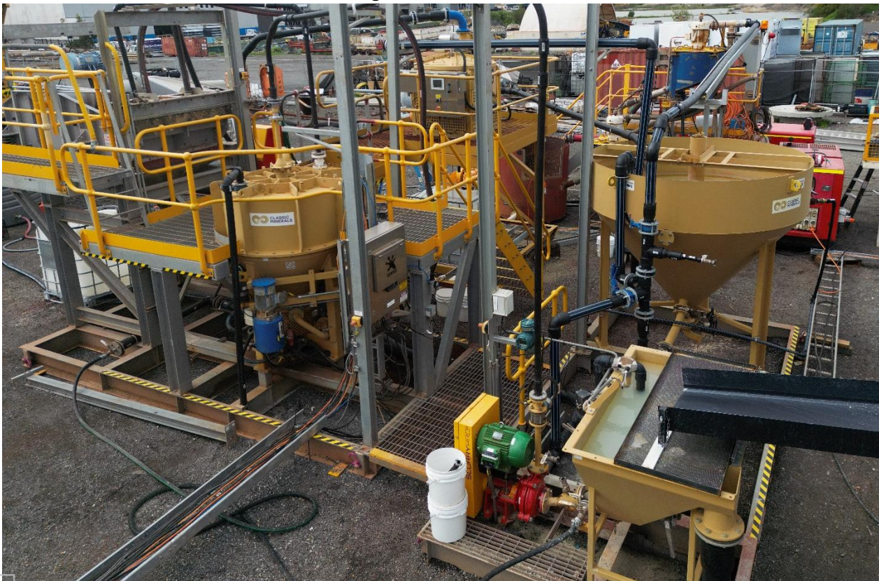
Figure 2: Gekko Pilot Plant
