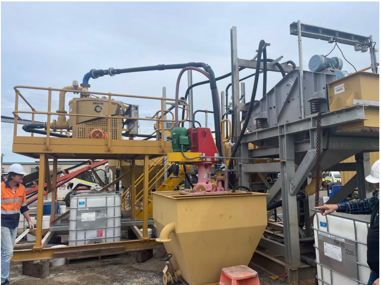
Figure 1: Gekko Pilot Plant
