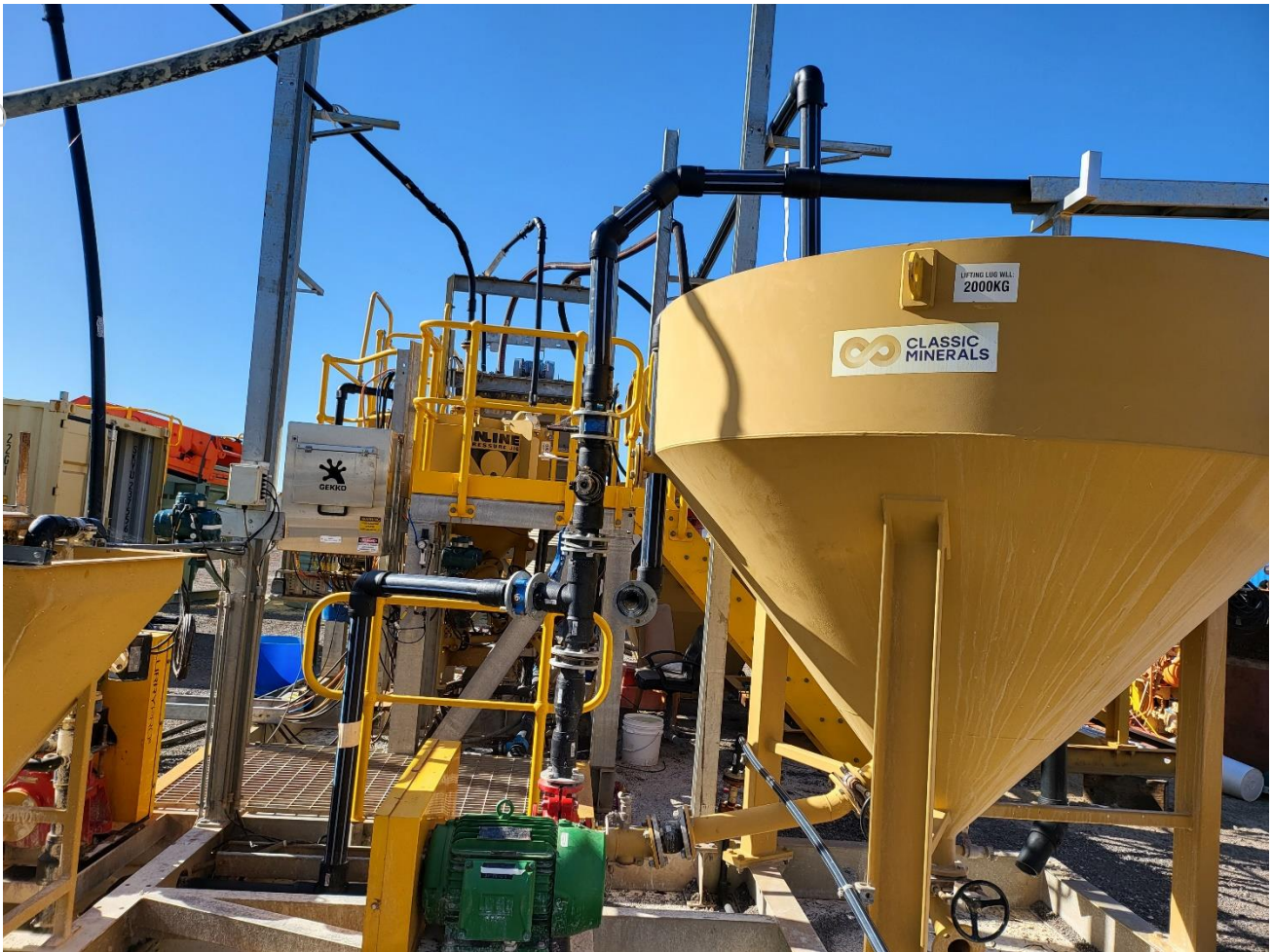
Figure 3, 4, 5, 6 & 7: Gekko Pilot Plant
