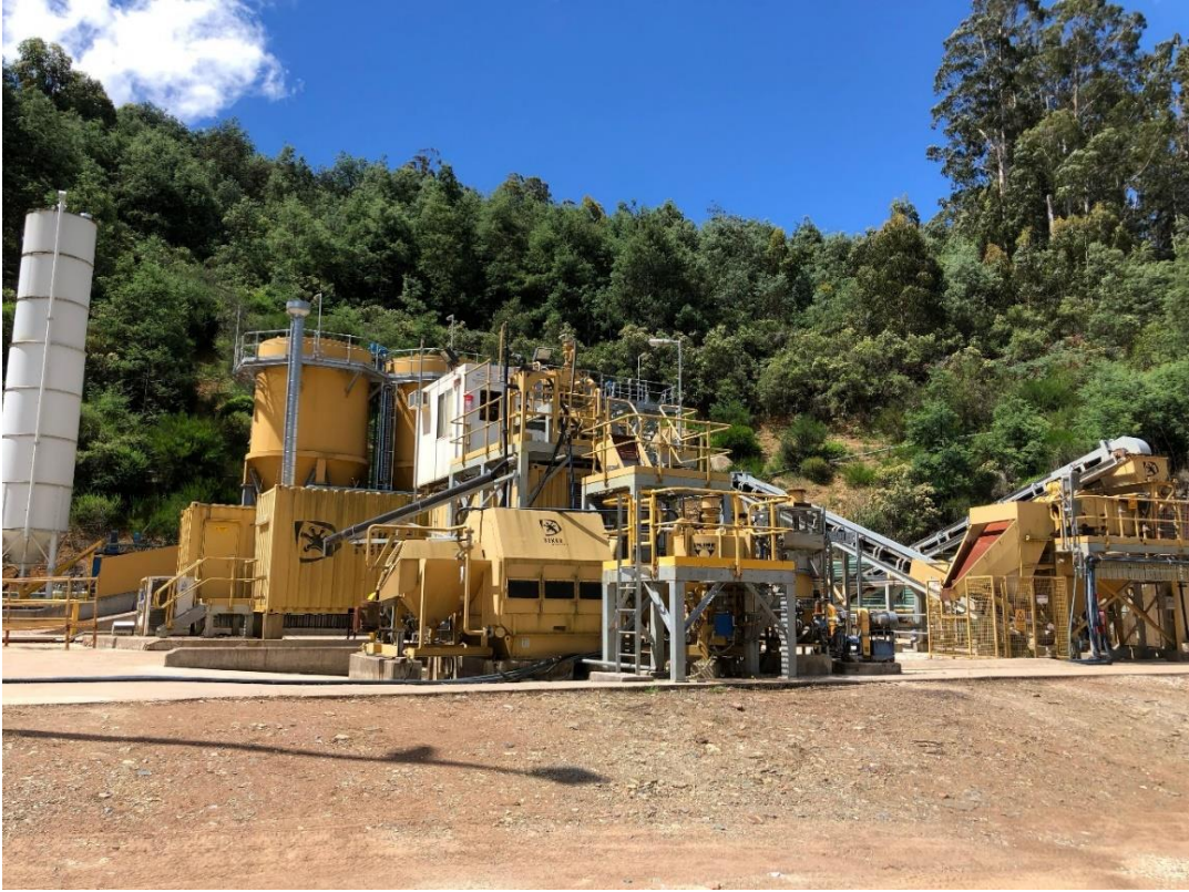
Figure 3: Gold processing plant at White Rock's Morning Star Gold Mine, NE Victoria
