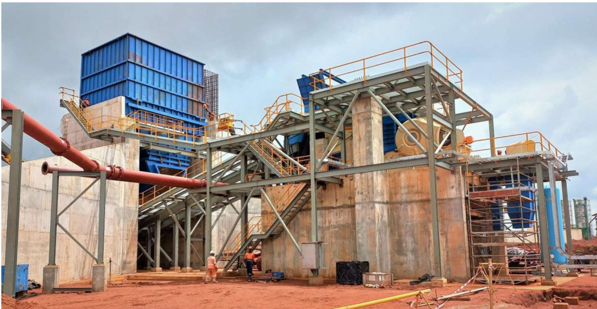
Figure 5 Crusher and ROM Bin
