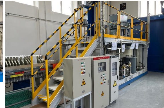
4. Leaching and Purification Module
