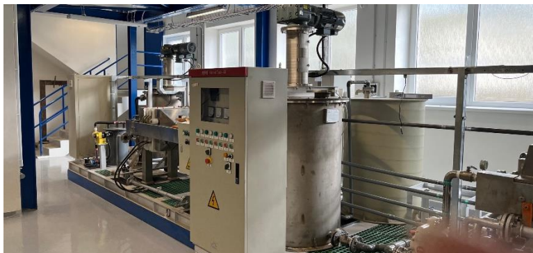
7. HPMM Dissolution, Deep Final Purification Module
