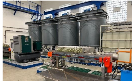
3. Post Magnetic Separation: Concentrate and Tailings Tanks and Filter Presses
