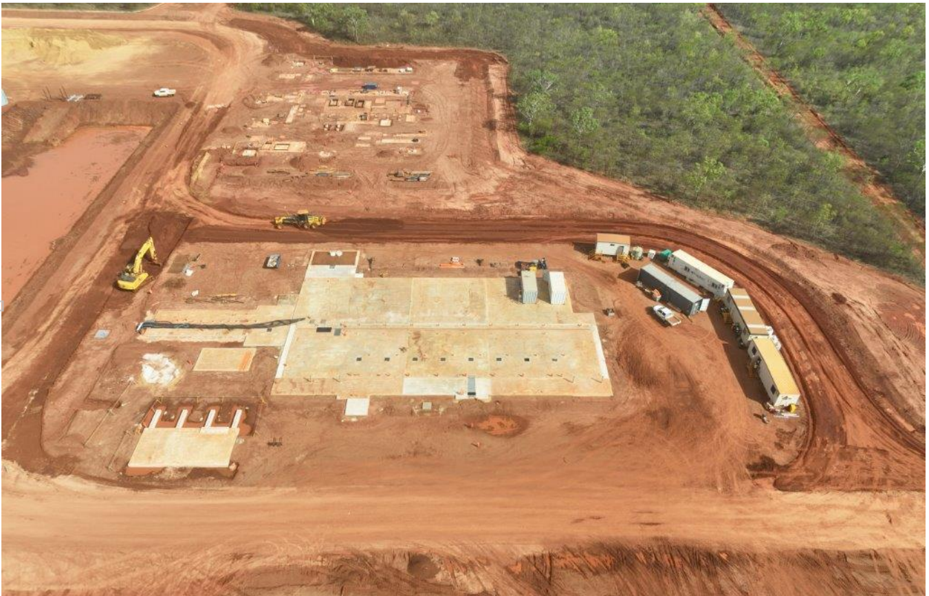
Image 4: Power Station concrete works completed ahead of installation by Pacific Energy Pty Limited
