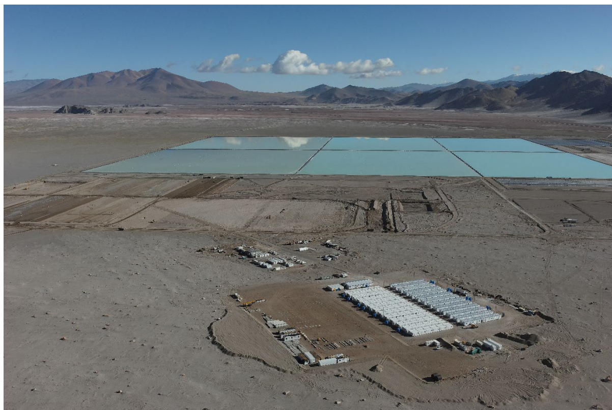
Figure 3: Sal de Vida Stage 1: Camp expansion (forefront), earthworks (centre), first 2 strings (background)
