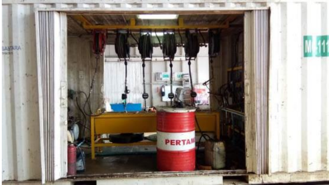
Figure 30 HV Workshop Lube container
