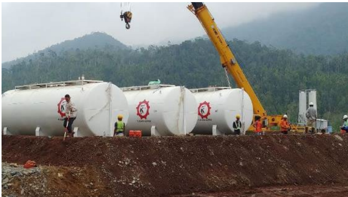
Figure 33. Example of 50kl fuel Storage Tanks – Nickel Mining Facility
