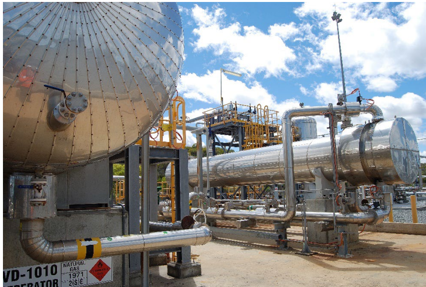
Figure 3: Arrowsmith Stabilisation Plant (ASP) Processing Facilities
