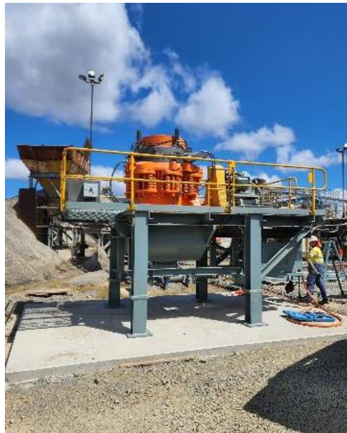
Figure 2 - Tertiary Cone Crusher for XRT Sorter Concentrate
