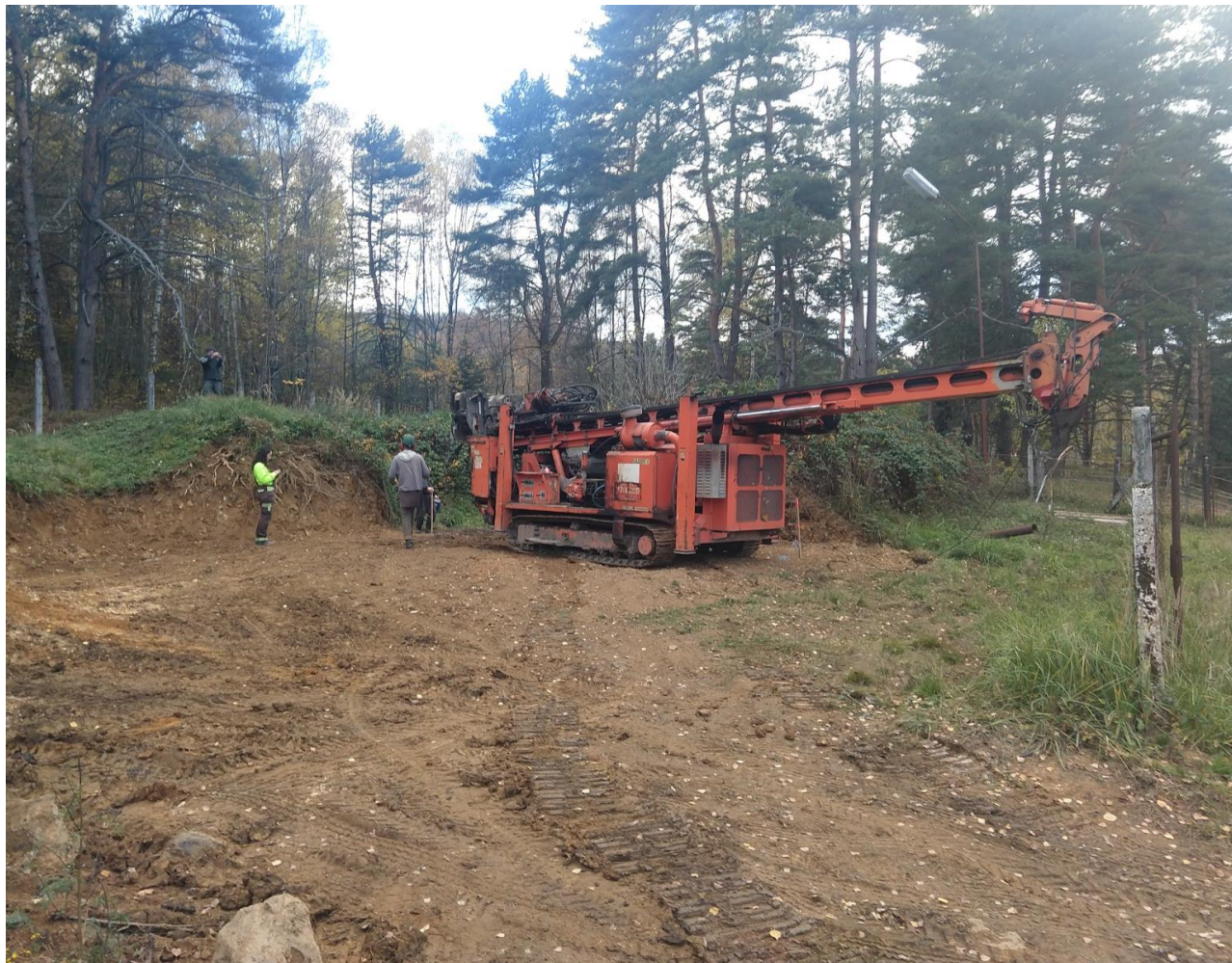
Figure 10: Diamond drill rig set up at the first target area, site preparation completed, location of drill hole SSD-01
