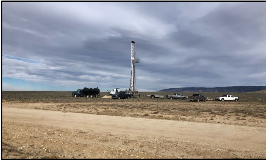
FIGURE 5: MUD ROTARY DRILL RIG OPERATING, ODIN ISR URANIUM PROSPECT, GDB WYOMING, USA
