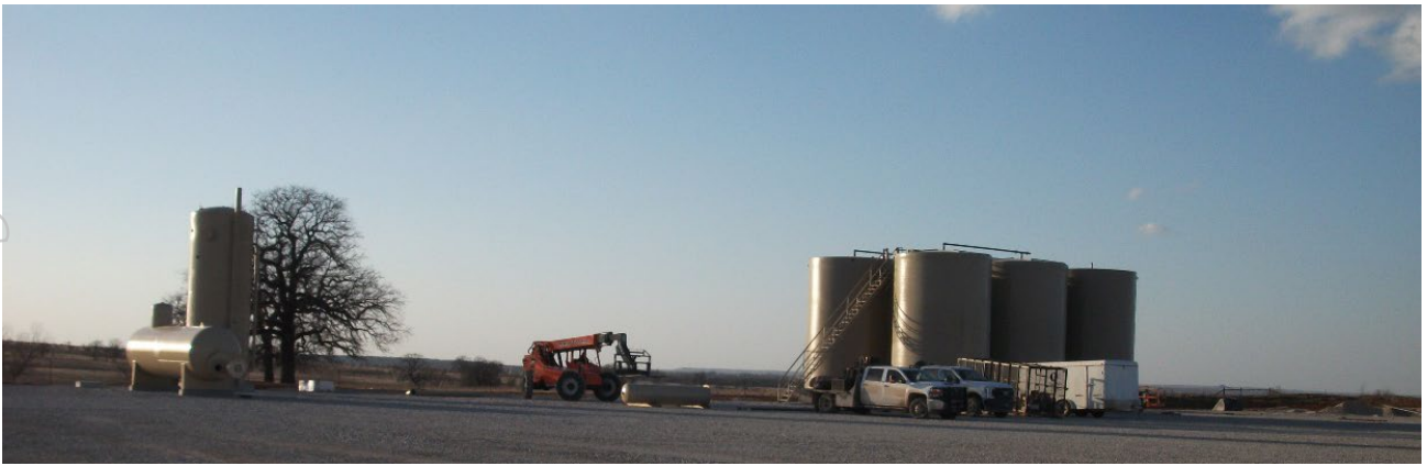
Figure 4. Rangers tank battery and separators
