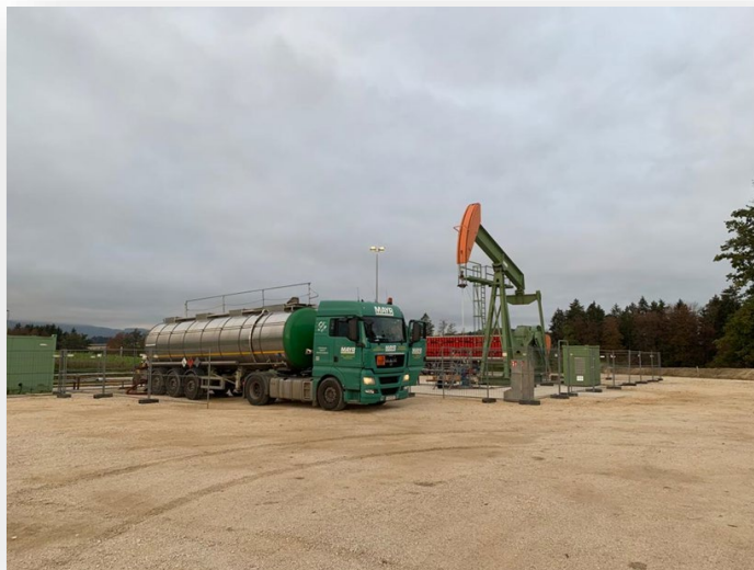
Oil Tanker offloading at Anshof-3 Location
