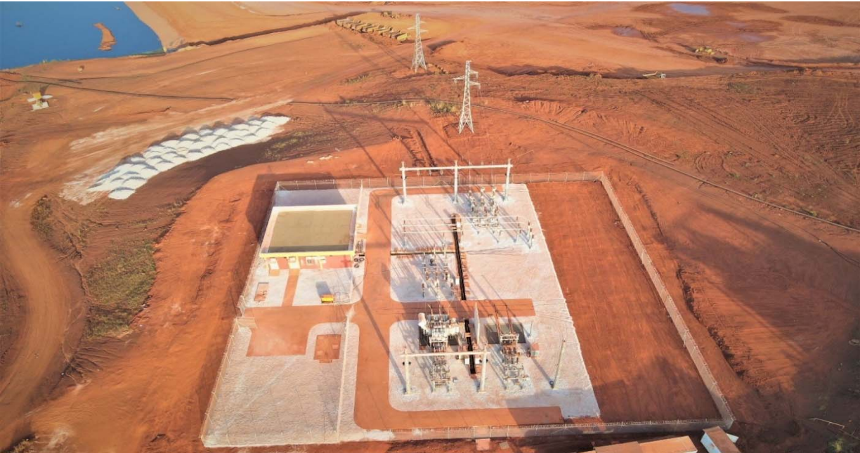
Figure 8: Abujar 90kV substation
