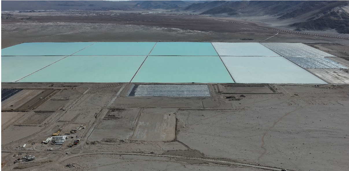
Figure 2: Sal de Vida Stage 1: First 2 string of ponds are 90% complete and carbonation plant development advances
