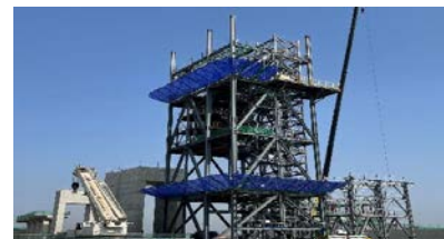
Figure 4: Acid Roasting Pre-Heater
