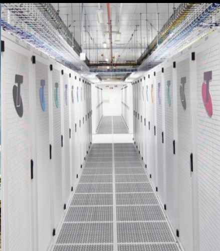
CIP: TELSTRA DATA CENTRE COMPLEX, CLAYTON, VIC
